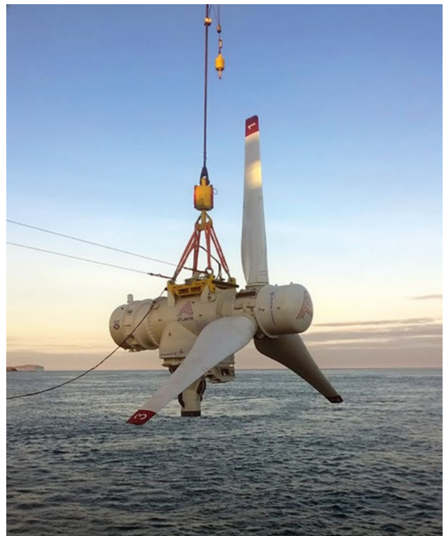
SIMEC Atlantis Energy turbine deployed in Scotland's Pentland Firth (Meygen project) Courtesy: Simec Atlantis Energy
